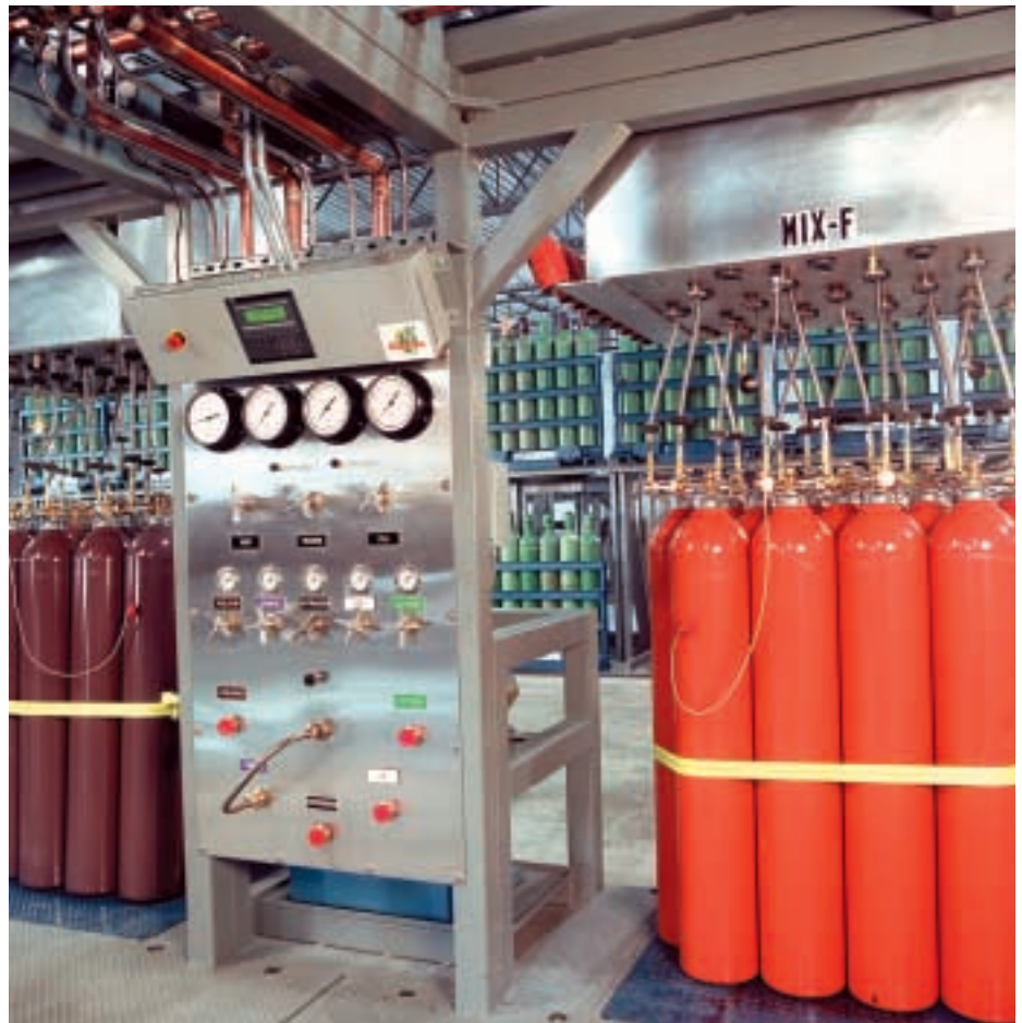
A Weldcoa gas filling station uses thermocouples magnetically attached to the canisters to monitor the progress of a fill. A gravimetric scale can also be used to update the program of weight changes during the fill.
